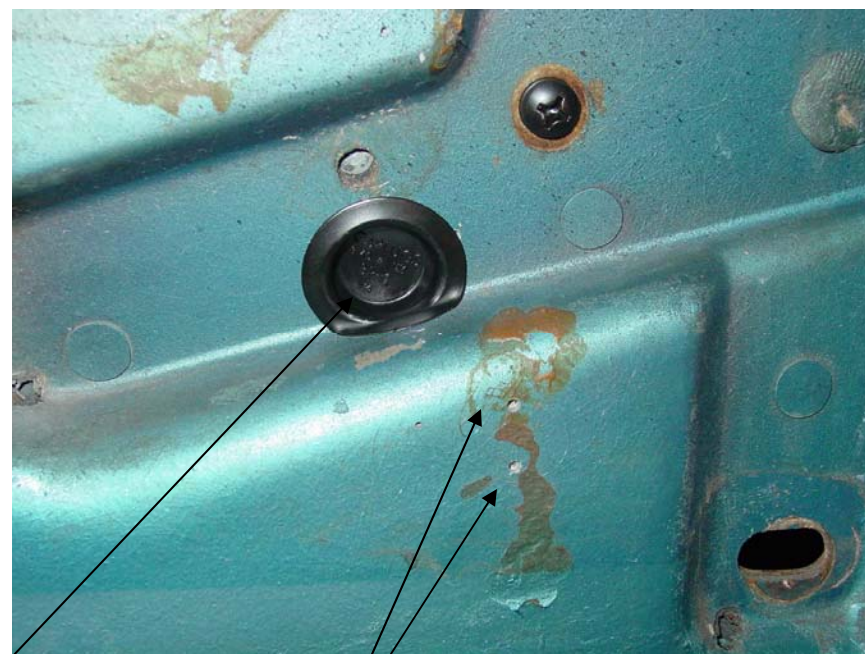
Used a very small drill bit to drill test holes to locate the sash stud at the front of the window. Probe with a thin wire to see where you are in the door.
